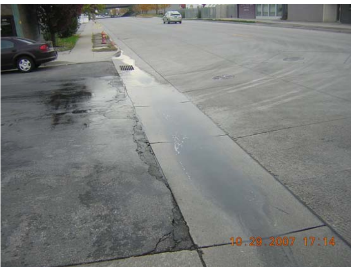
Soapy, dirty water flows in the gutter near a major company that was repeatedly discharging their wastewater into the storm drain.
